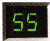
Displays Supply Duct Air Temperature
